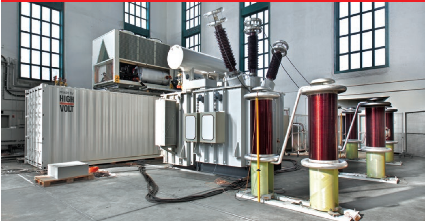
Fig. 1 Transformer test system based on static frequency converter, type WV 2000-4000/170
